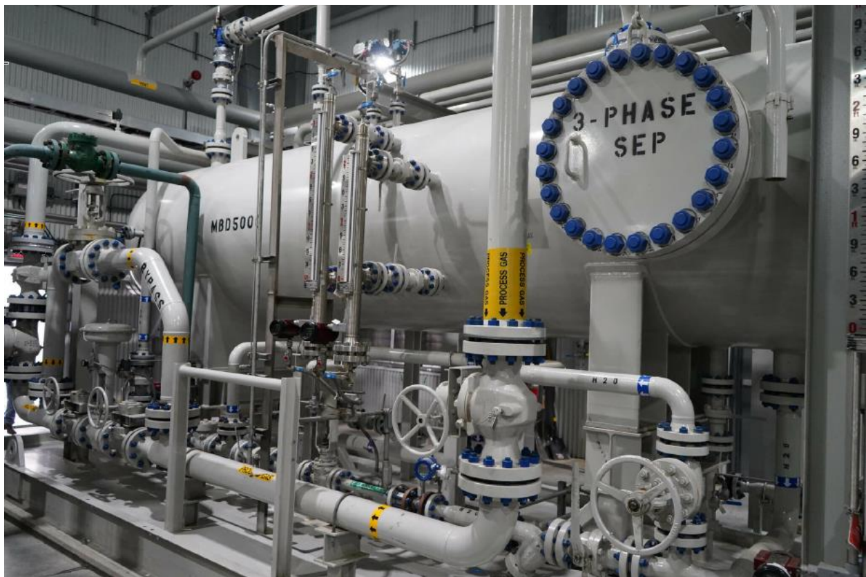
Natural gas processing equipment is seen at Furie Operating Alaska's central processing facility in Nikiski, Alaska, on Wednesday, July 10, 2024. (Jake Dye/Peninsula Clarion)
